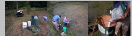
Equipment used to mix dry alum with water: pump and 55-gallon drum
